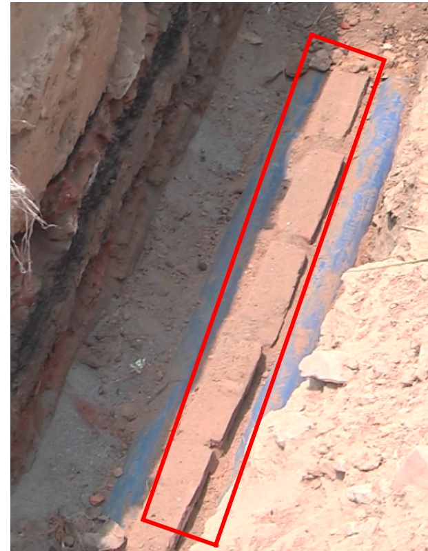
Circuits running parallel with brick padding
