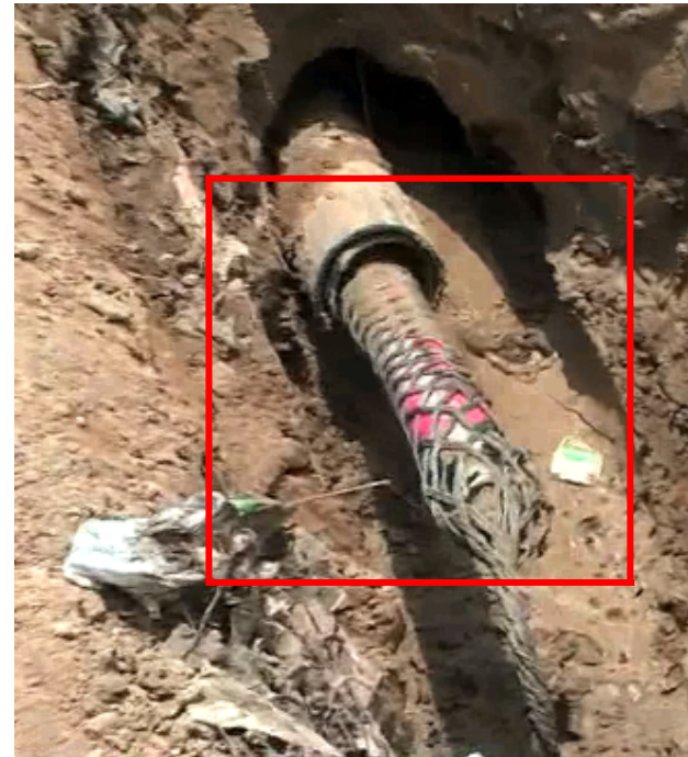
End of the cable
